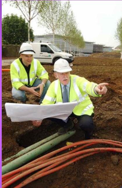
Oil Filled Cables
